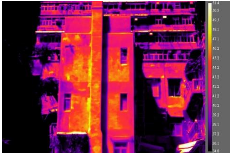
Figure 4 A typical thermogram with defects (Acknowledgement: Fugro Technical Services Limited)
